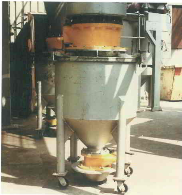
WASTE COLLECTION BINS USED BY A MAJOR BREWER. 300mm DISC VALVE IS FITTED TO TOP AND 150mm DISC VALVE FITTED TO OUTLET
