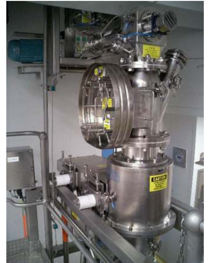
A custom built Kek 220 Cone Mill in a pharmaceutical process line
